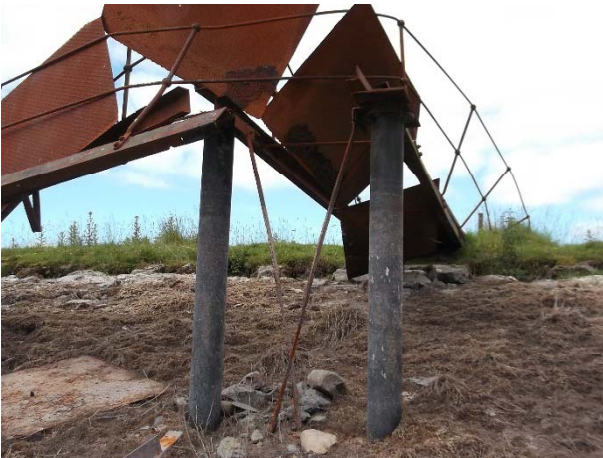
Valve tower access
