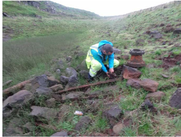
Overflow & Outlet (vandalised)
