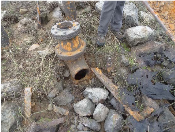
Overflow & Outlet (vandalised)
