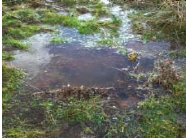
Possible leakage (d/s dam)
