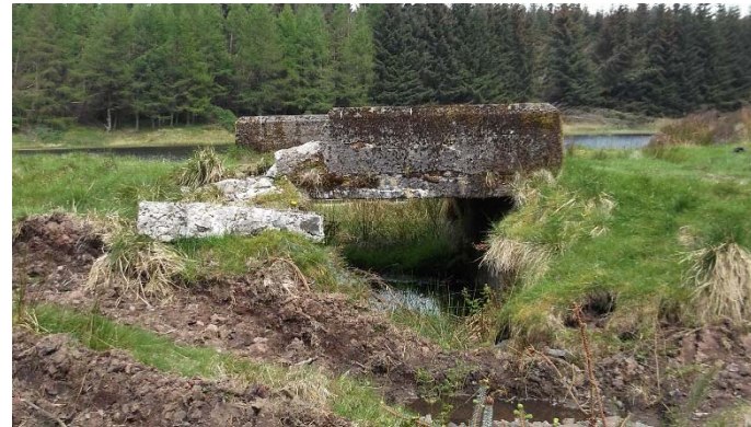
Damaged Spillway Crossing
